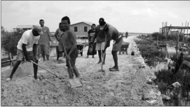
San Mateo residents build roads with supplies purchased by Ole Miss students.
